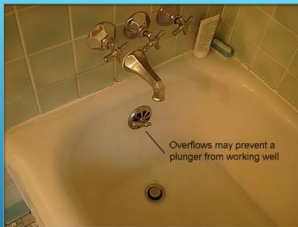
405.7 Design of overflows. Where any fixture is provided with an overflow, the waste shall be designed and installed so that standing water in the fixture will not rise in the overflow when the stopper is closed, and no water will remain in the overflow when the fixture is empty.
