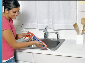
405.5 Water-tight joints. Joints formed where fixtures come in contact with walls or floors shall be sealed.
