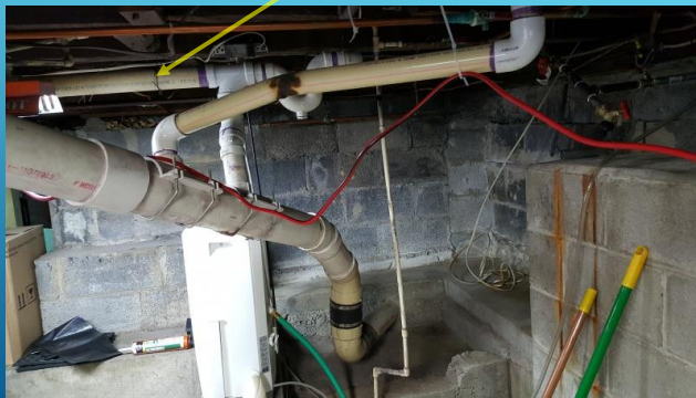
One Hanger on the drainage system
