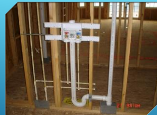
406.2 Waste connection. The waste from an automatic clothes washer shall discharge through an air break into a standpipe in accordance with Section 802.4 or into a laundry sink. The trap and fixture drain for an automatic clothes washer standpipe shall be not less than 2 inches (51 mm) in diameter. The fixture drain for the standpipe serving an automatic clothes washer shall connect to a 3-inch (76 mm) or larger diameter fixture branch or stack. Automatic clothes washers that discharge by gravity shall be permitted to drain to a waste receptor or an approved trench drain.
