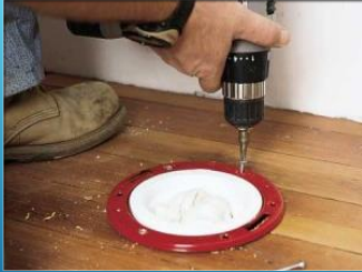
405.4.2 Securing floor outlet fixtures. Floor outlet fixtures shall be secured to the floor or floor flanges by screws or bolts of corrosion-resistant material.
